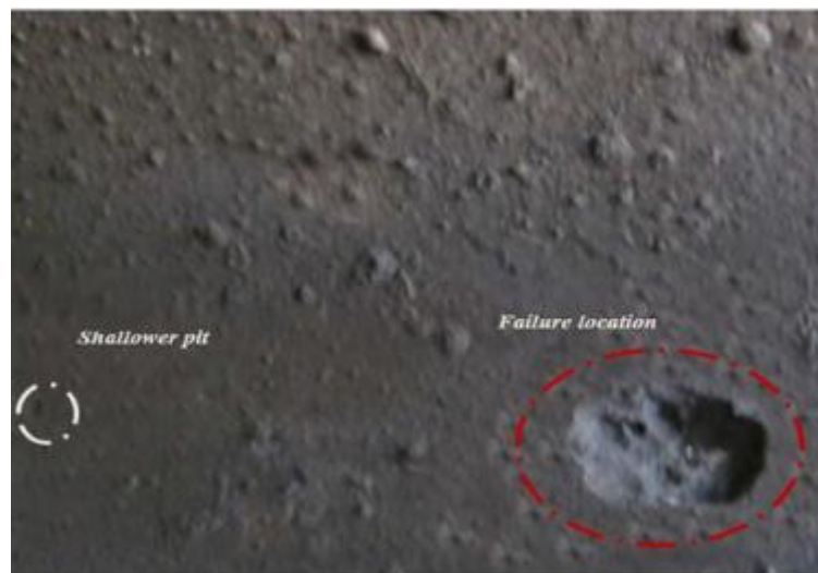
Figure 2.2: Pitting corrosion at internal surface of pipeline (Mansoori et al., 2017)
