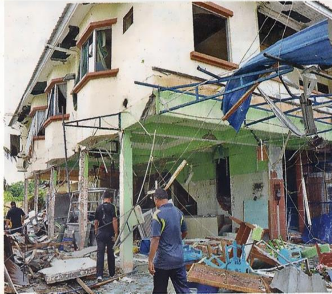
Building that housed the eatery and confectionary shop damaged in the explosion
