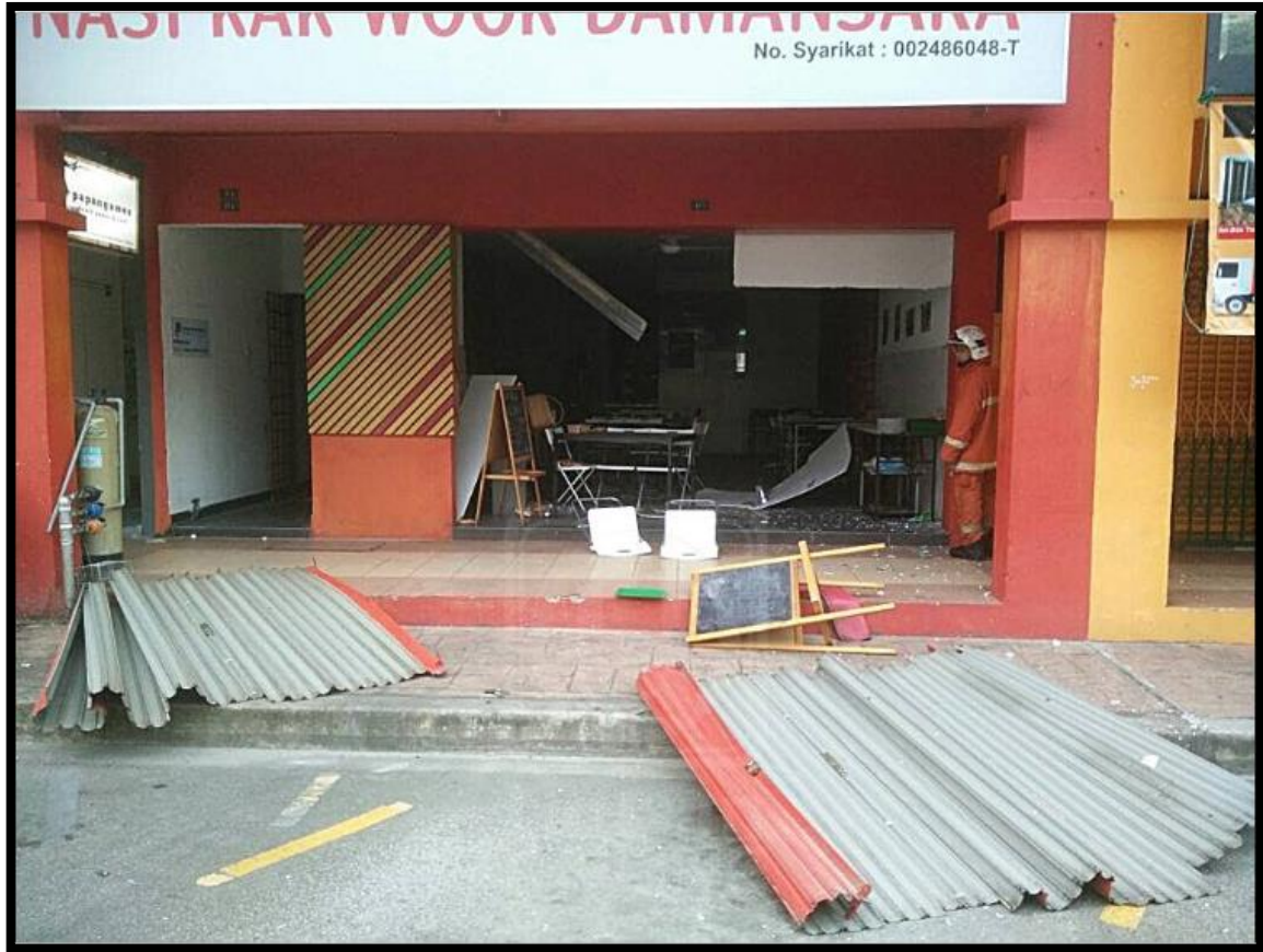
Figure 1.2: The damage and losses of the restaurant due to explosion.
