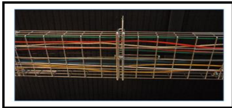
Figure 2.2: Overheat Cable Tray (Lensu, 2013).
