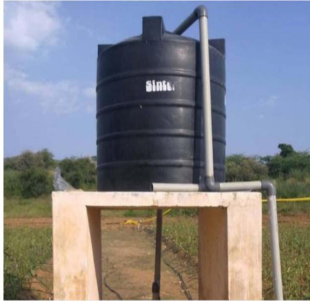
Figure 2.1: A 1000 litres capacity drum mounted on a concrete form
