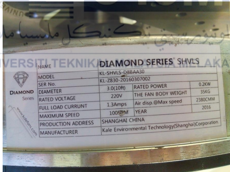
Figure 3.4 : Nameplate of the HVLS fan
