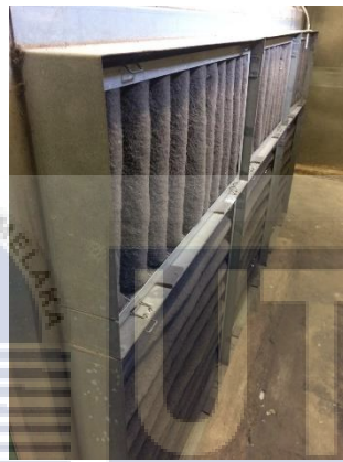
Figure 4-14: AHU air filter
