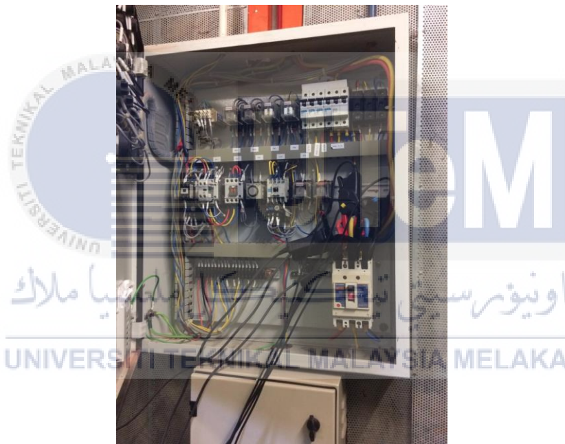
Figure 3-7: Power Logger at First Floor AHU Distribution Board
