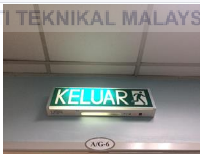
Figure 4-20 1 × 13W T5 Fluorescent Exit Sign Light
