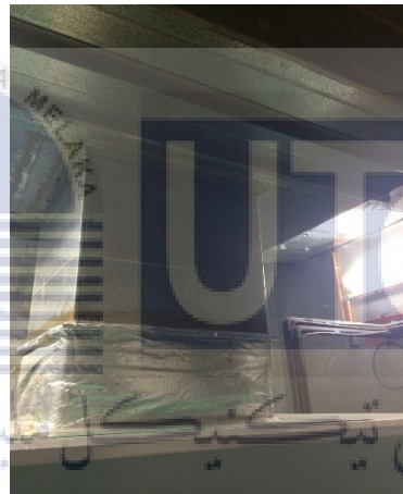
Figure 4-5: AHU Evaporator Coil
