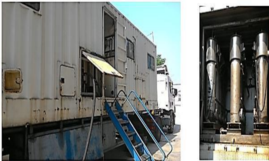
Figure 2-3 : Online Mobile Insulating Oil Reclamation Plant: (left) Mobile Truck; (right) Column Tanks Filled with Adsorbent [1]
