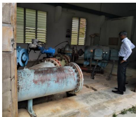
Figure 1.1 Site visit at the pump station
