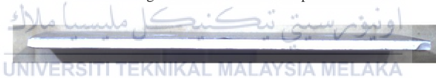
Figure 4.7: Crack Tile Sample
