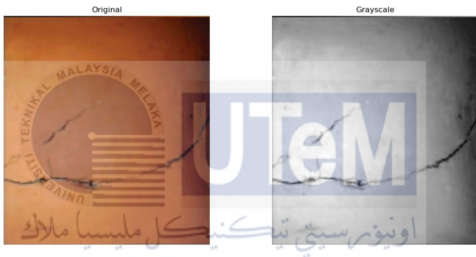
Figure 4.3 Original Image [36] and Grayscale Image for Crack 9
