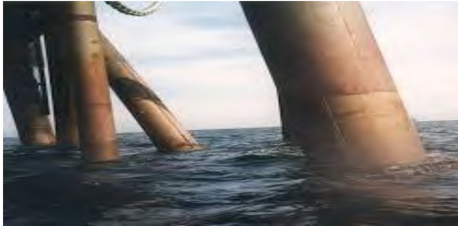
2.3(a) Corrosion of Copper
