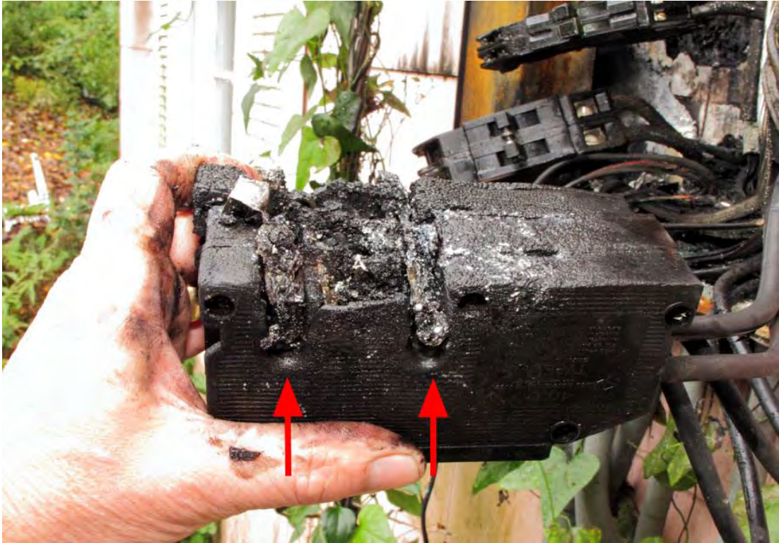
Figure 1.2: Example of broken component circuit breaker and cause a short circuit
