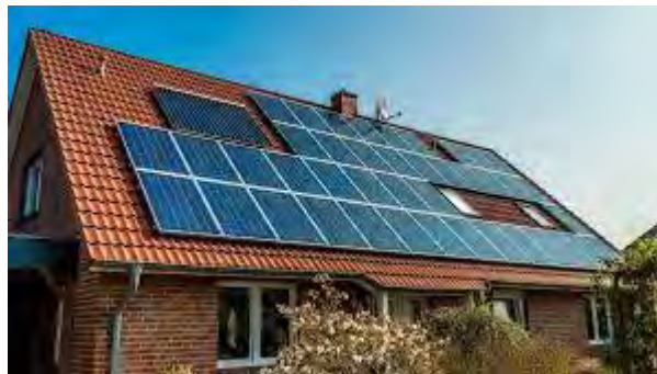
Figure 1.1: The Fixed Solar Panel Mount On The House
