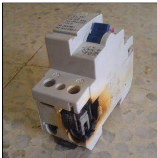
Figure 1.1: Burning ELCB caused by a short circuit
