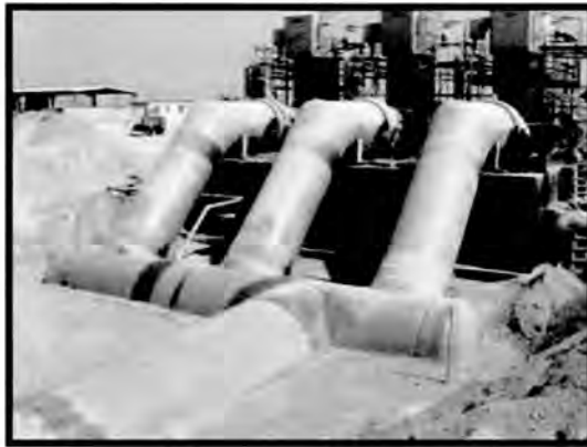
Figure 1.2: FRP piping system applied in industry
