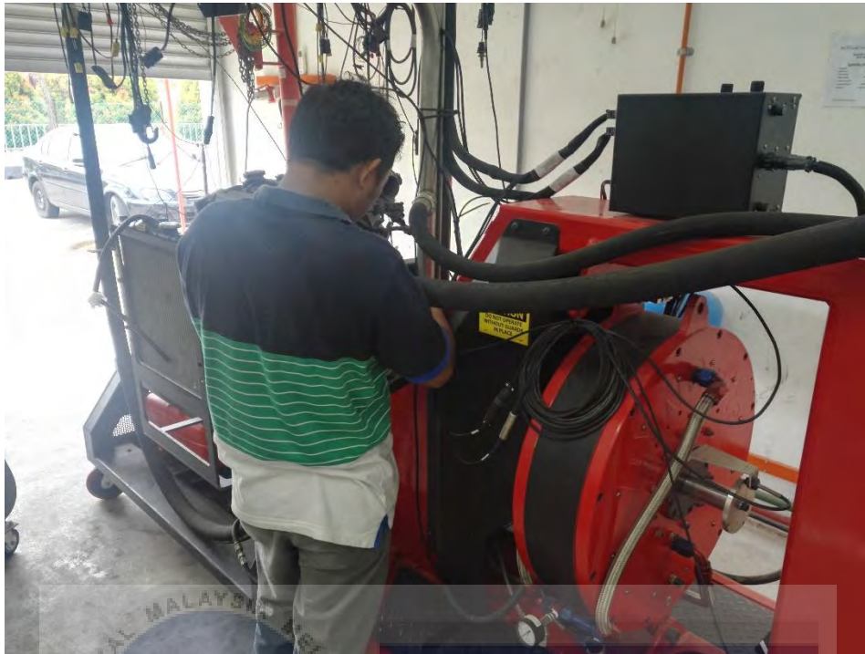
Appendix D: Assistant Engineer change the Electronic Controller Unit of the engine
