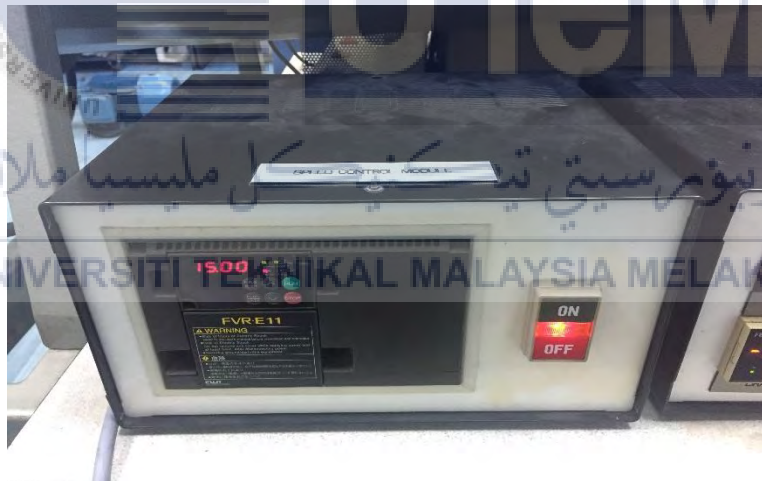
Figure 3.7.3 Speed control module is being set at the frequency of 15Hz
