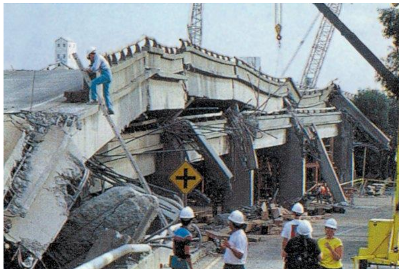
Figure 2.1: Cypress Freeway that collapsed during the 1989 earthquake
