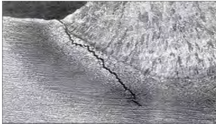
Figure 2.1: Fatigue crack in structure.
