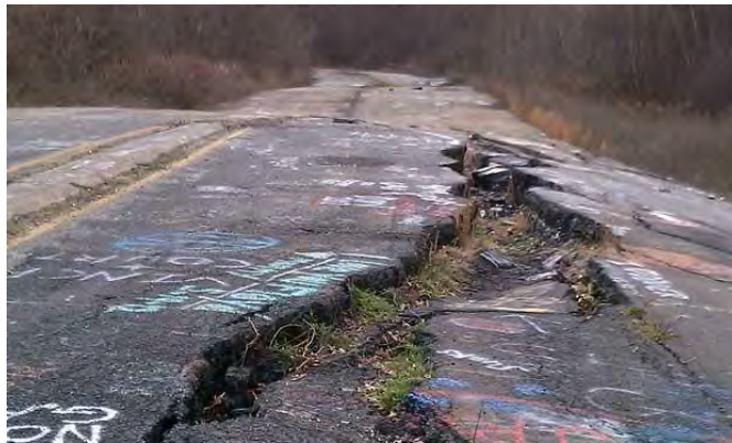
Figure 1.2.1: An example of road irregularity.
