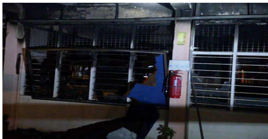
Figure 1.3: Shows the position of fire extinguisher
