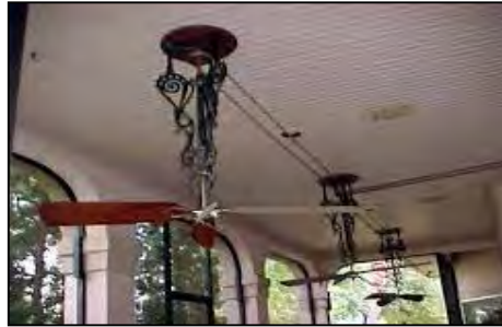
Figure 1-3 : Belt driven ceiling fan
