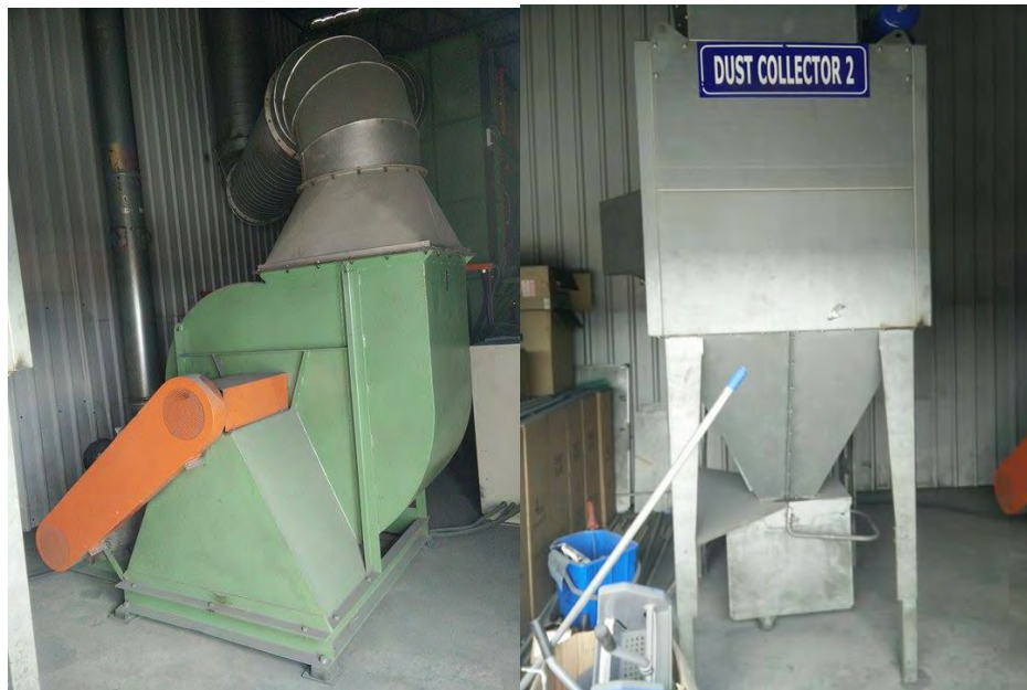
Figure 2.1: Current dust collector system in CTRM
