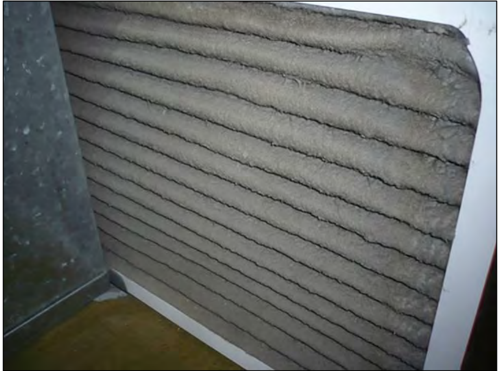
Figure 2.3: Bad AHU air filter.
