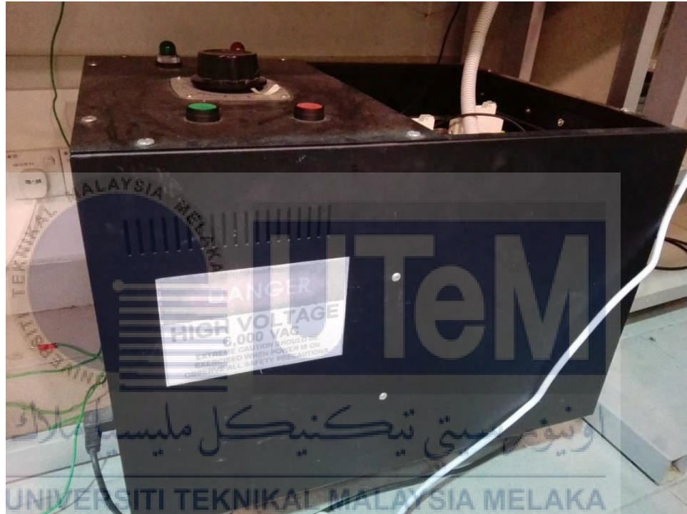
Figure 3.5: The variable single-phase high voltage transformer 0-6kV.
