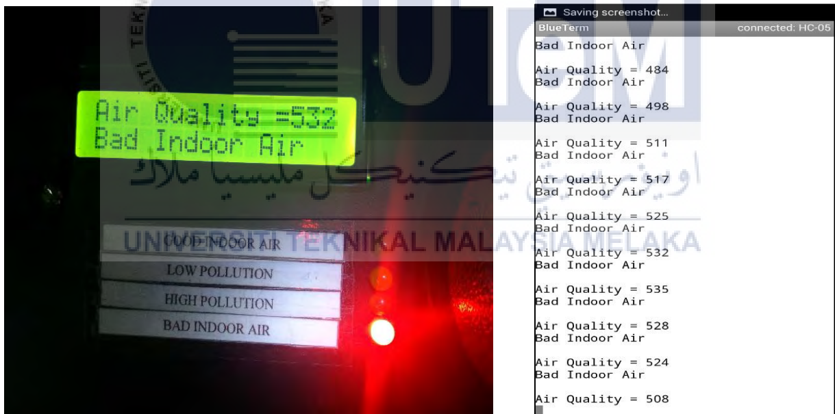
Figure 4.16: The condition change to “Bad Indoor Air” after 6 second and printed out the condition on the LCD and Smartphone application.
