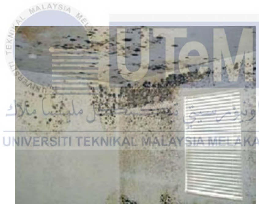
Figure 2.3: Mould causes by leaking pipes [20].
