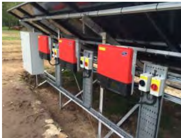
Figure 2.3: Grid-connected Photovoltaic inverter.
