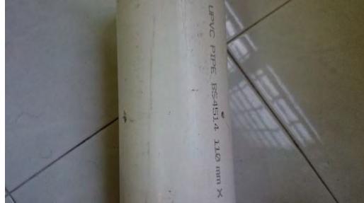
Figure 3.6: Hole on the pipe surface
