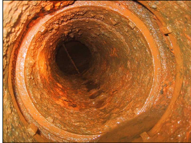
Figure 1.1: Caustic Corrosion (Lesley.B, 2016)
