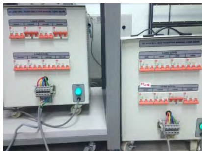
Figure 3.6: Resistive and Inductive load bank.
