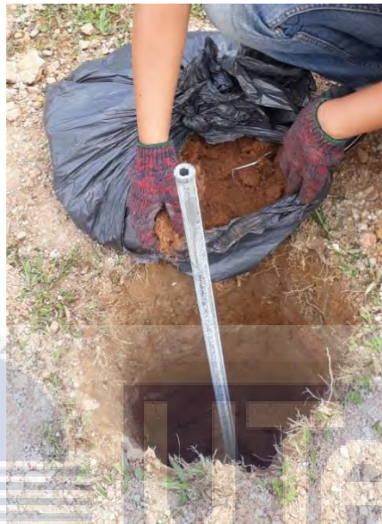
Figure 3.5: Galvanized steel ground electrode (hollow rod) at testing site.
