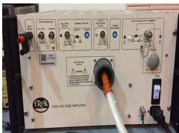
Figure 3.12: High voltage amplifier
