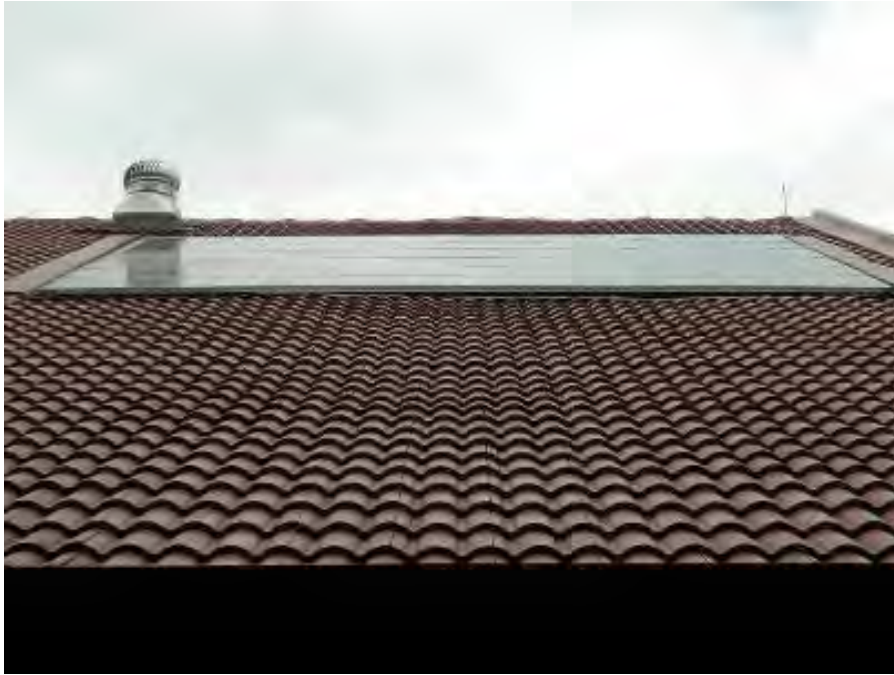
Figure 2.2: A 4.3kWp GCPV on the rooftop of the house at Bukit Beruang[19].
