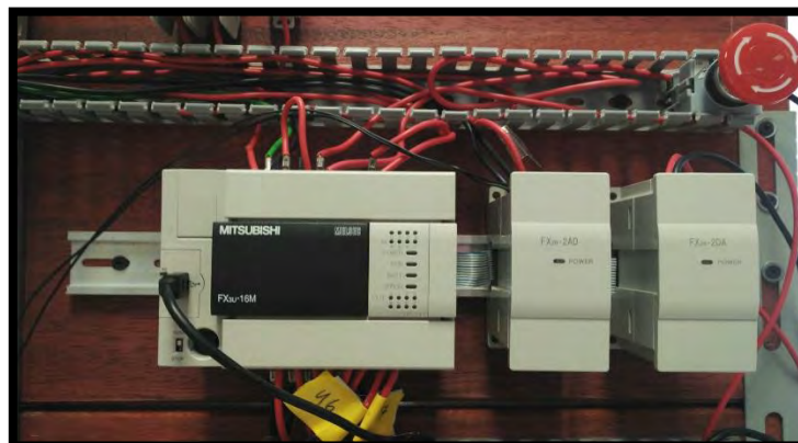
Figure (g): PLC interface.
