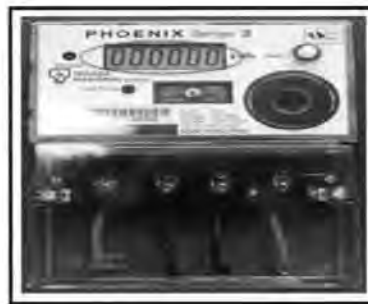
Figure 2.1: The LCD display shows meter reading is 0 kWh
