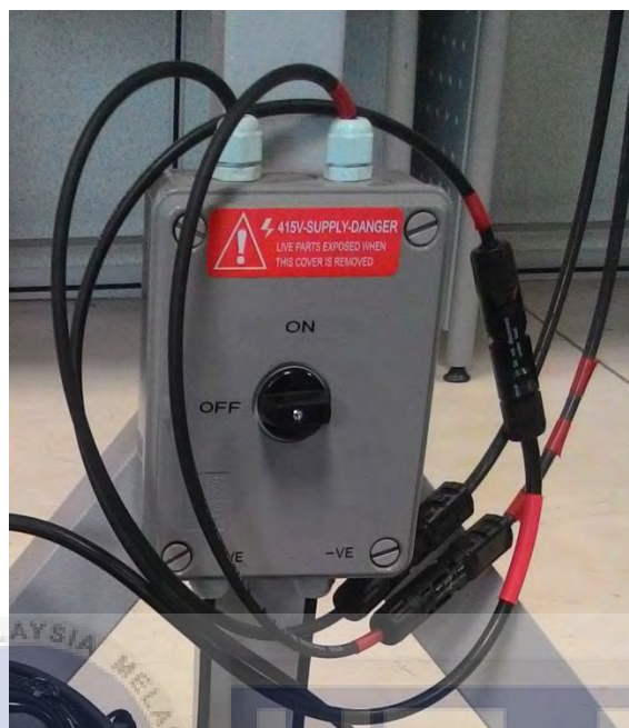
Figure 3.9: Part of isolator
