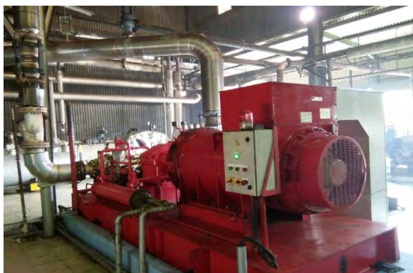
Figure 4.2: Generator at Palm Oil Factory
