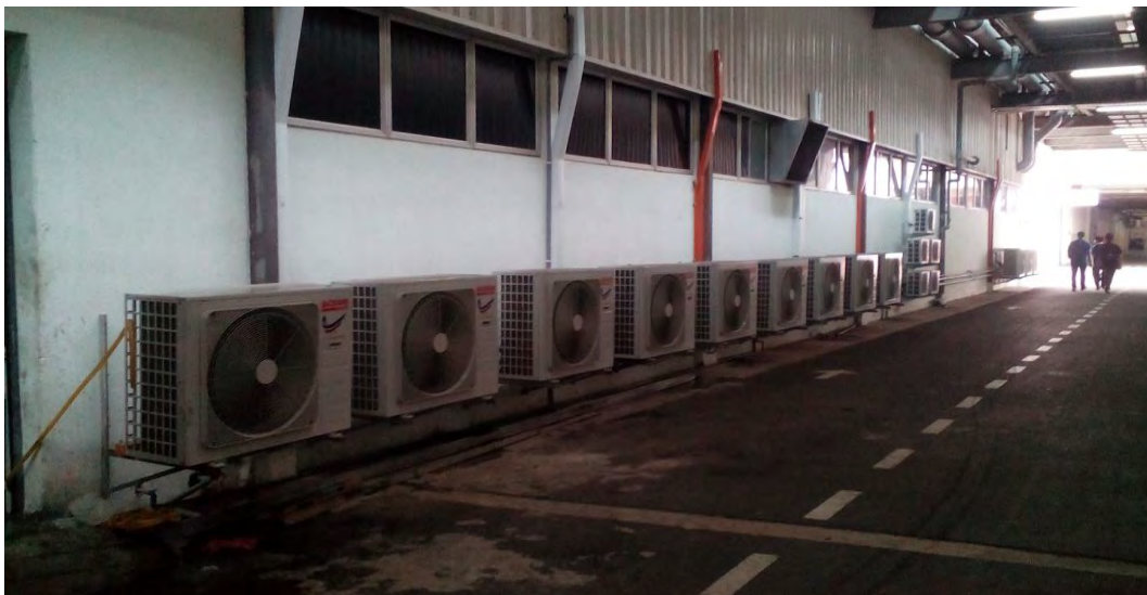
Appendix E: Split unit used at Factory 1
