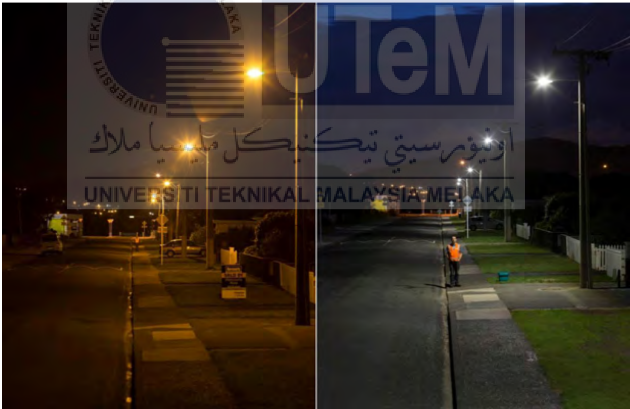
Figure 2.8 Smart street lighting
