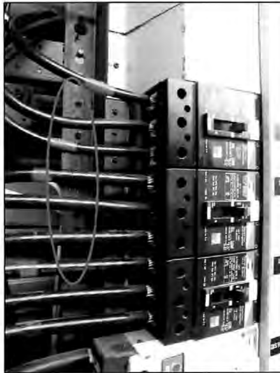
Figure 2.3 Electric junction box badly corroded only four years after a new residence was completed.
