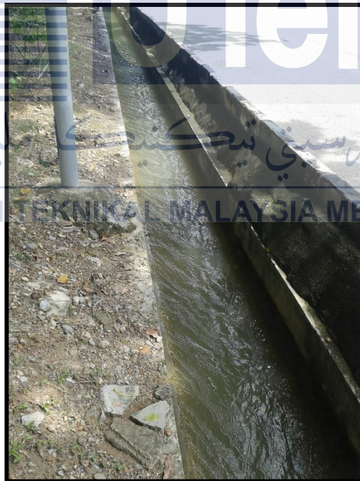
Figure 4.0: First checkpoint of drainage.
