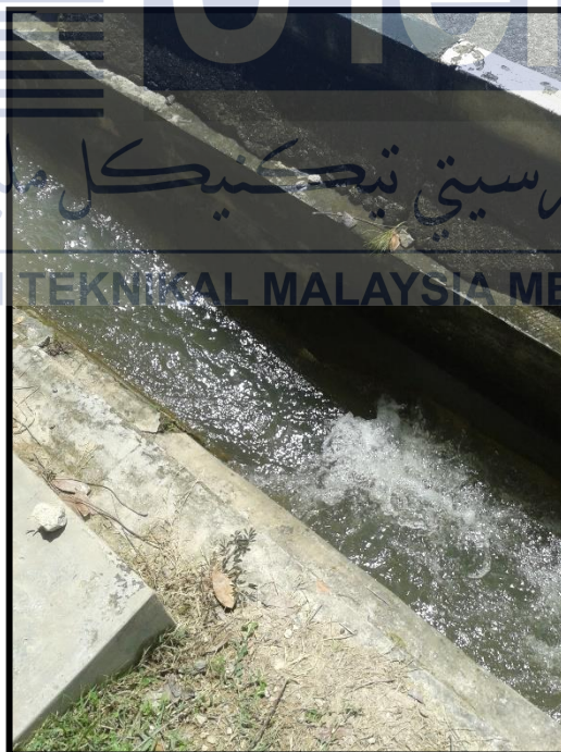
Figure 4.2: Third checkpoint of drainage.
