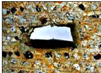
Figure 2.1.1: Holes in the walls (Chatfield 2005)
