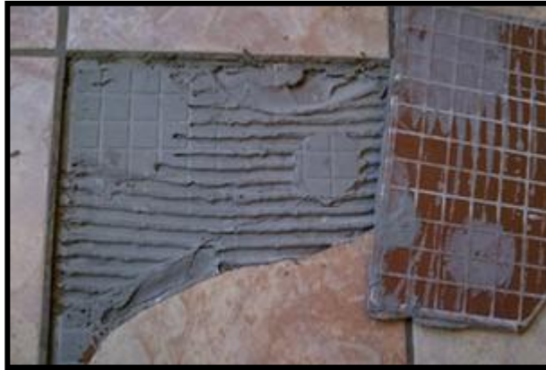
Figure 1.3 Ceramic tiles with cement failures.
