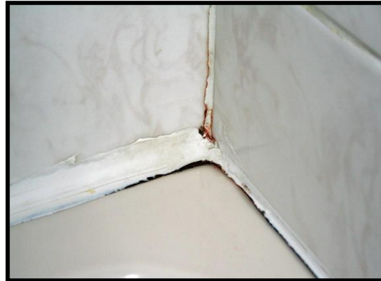
Figure 1.4: Failures of silicon glue
