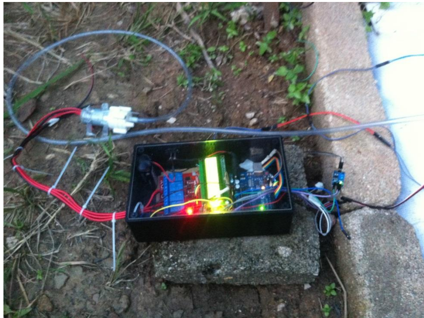
Figure 3.22 : Setting the controller
