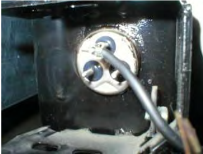
Figure 1.4: Compressor for air-conditioner that does not have terminal markings (Brand: Nordyne, Model: FS3BA-018KA)
