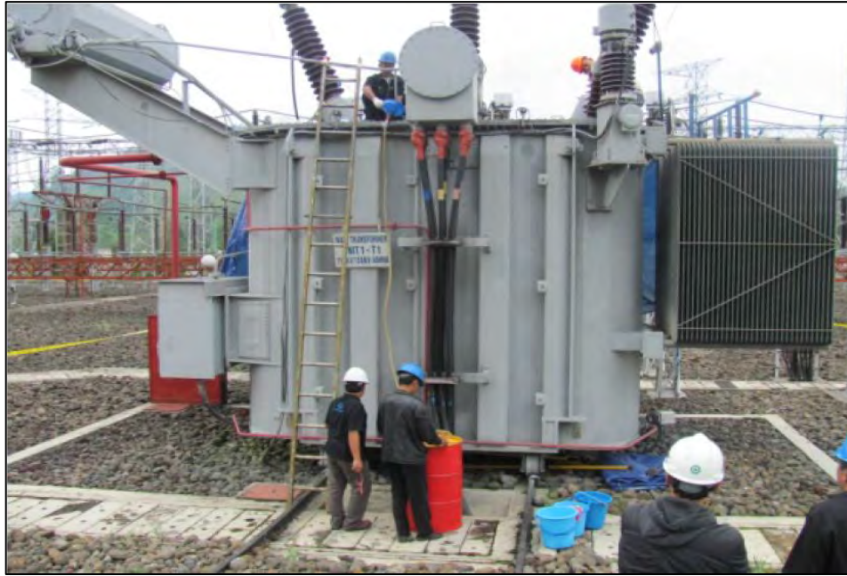
Figure 2.1: Power transformer rating of 40MVA is under maintenance Source: Purwadi et al. (2011)
