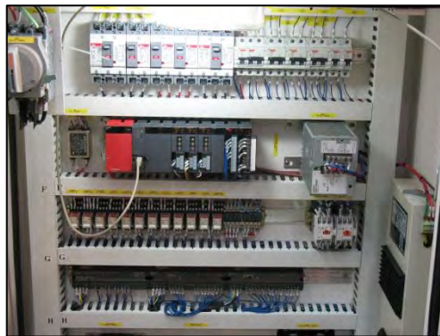
Figure 2.1: MITSHUBISHI PLC Panel
