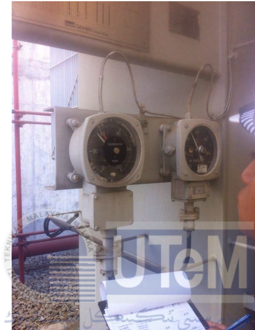
Figure 3.6: Auxiliary Transformer Temperature Gauge Meter
