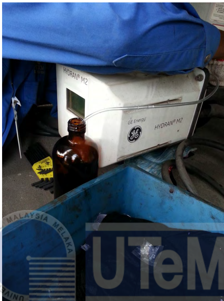
Figure 3.4: A Small Hose is Used to Collect the Oil Sample from The Drain Pipe Outlet
