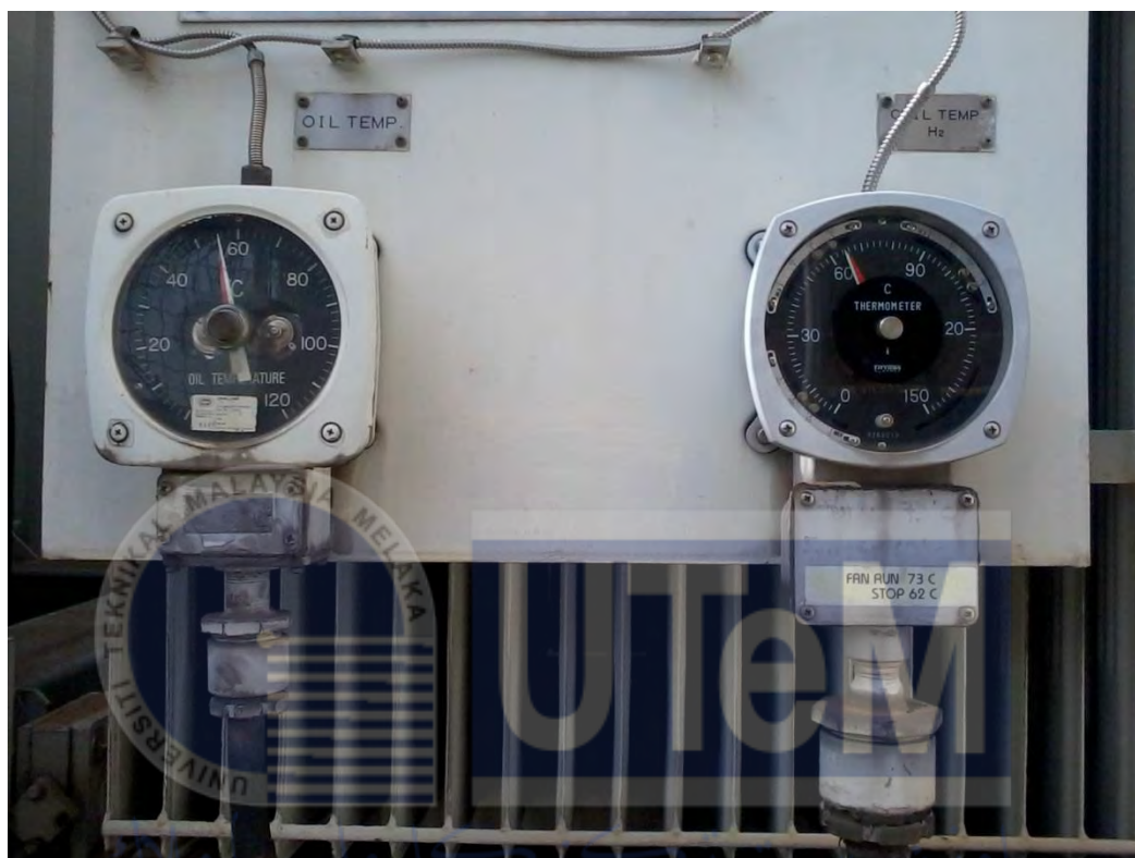
Figure 3.5: Generator Transformer Temperature Gauge Meter
