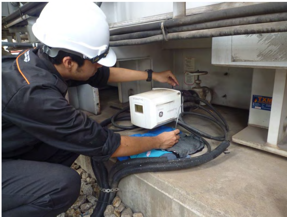
Figure 3.2: Oil sampling of Trasnformers by TXM Services Sdn. Bhd
