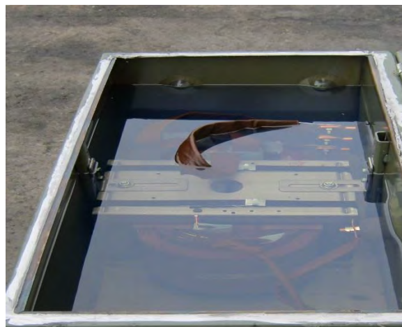
Figure 2.2: Insulating oil in an electrical power transformer [13]
