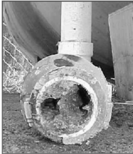
Figure 2: Blockages in Drain Pipe (Source: MMS, 2004)
