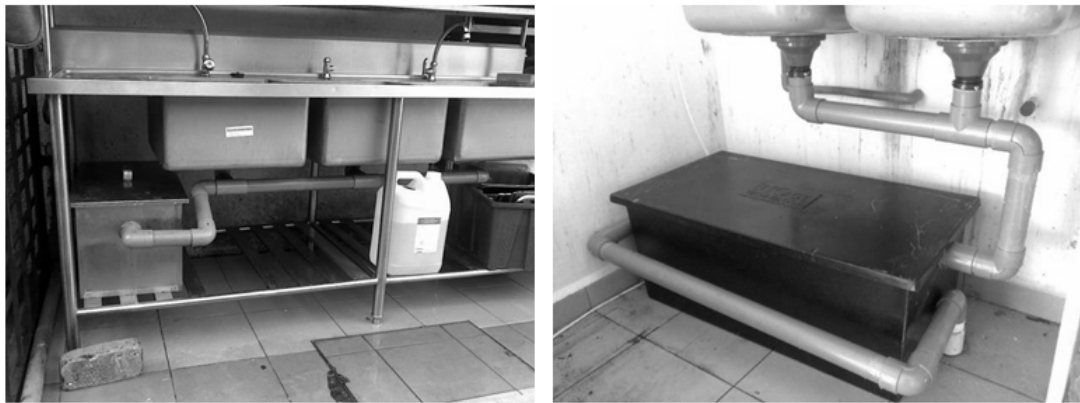
Figure 1: Example of Existing Grease Trap (Source: Lakasa, 2006)
